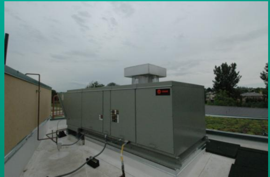
High Efficiency HVAC
