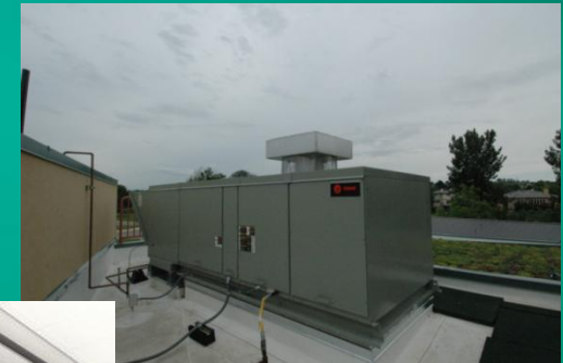
High Efficiency HVAC
